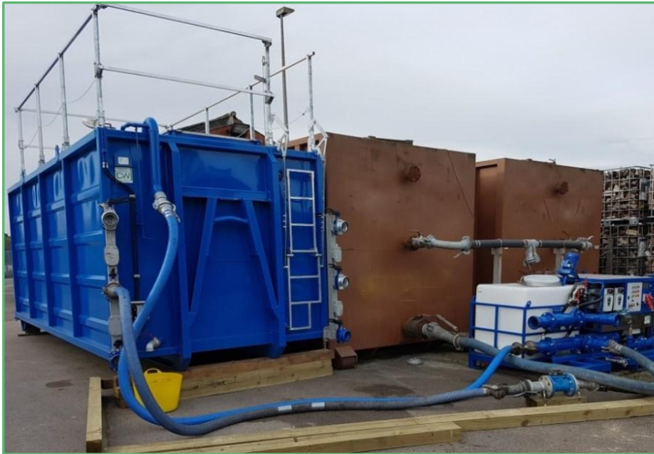
Above: STU set up with clients twin storage tanks and polymer dosing pump.
